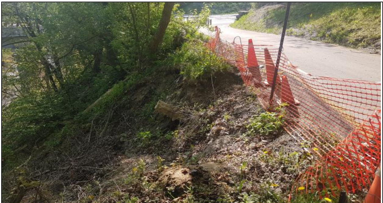
Figure 2. Slope crest with view of bare and unvegetated erosion scour on the slope crest facing east towards the Main Street South roadway.
