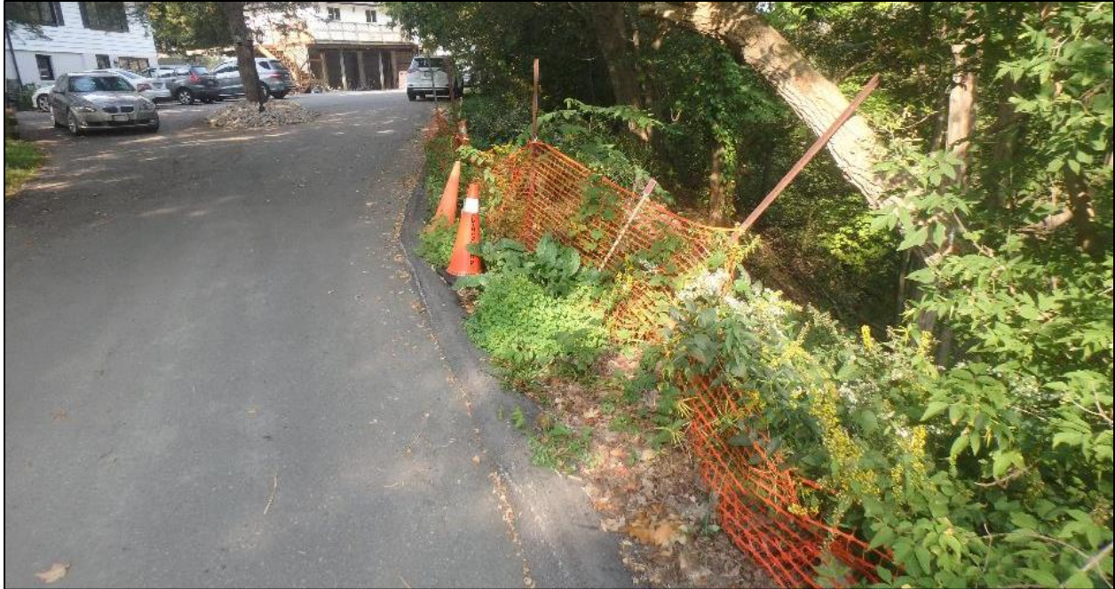
Figure 1. View of tableland conditions facing west; the erosion scour (surrounded by orange safety fencing) has grown in size since the initial inspection.
