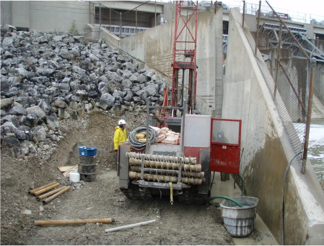
Figure 3 Claireville Dam wing wall settlement investigation.
