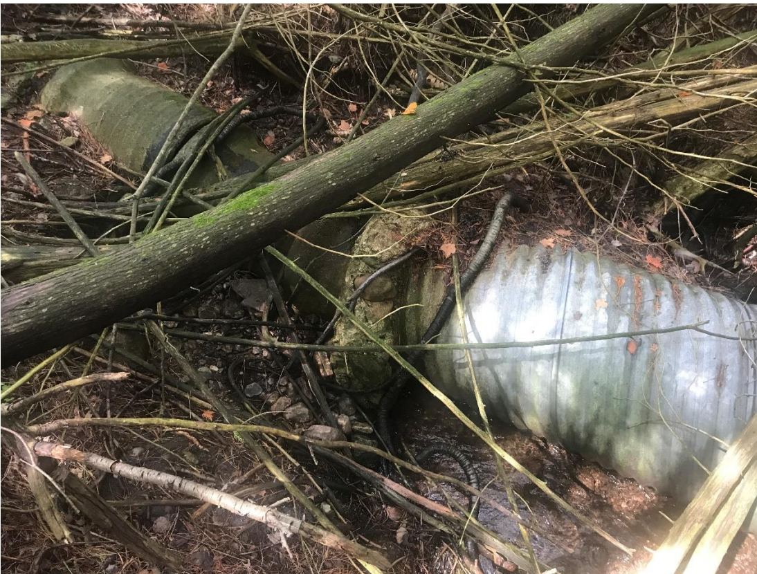
Figure 4 Failed spillway pipe at Glen Haffy Fly Fishing Upper Dam
