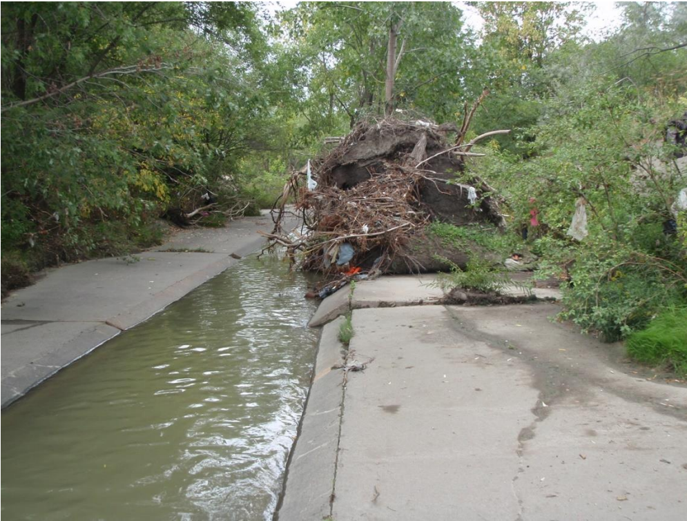
Figure 13 Partially blocked flood control channel at Black Creek.
