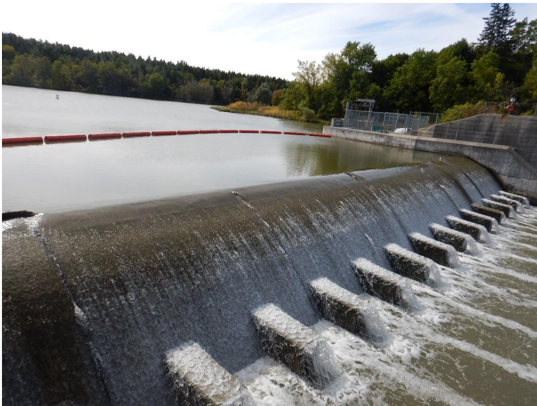
Figure 9 Milne Dam's spillway is too small for extreme floods and requires upgrades to withstand overtopping.
