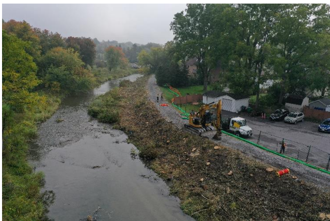
Figure 16 Bolton Berm repair as seen from drone survey (2020).
