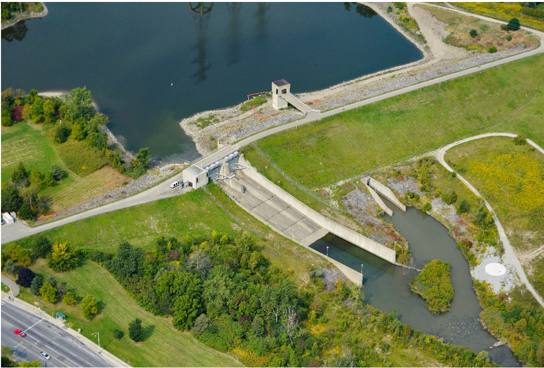
Figure 1 G. Ross Lord Dam carries the highest potential risk of any TRCA dam based on risk to life and property. G. Ross Lord Dam's EPP was finalized in 2019.
