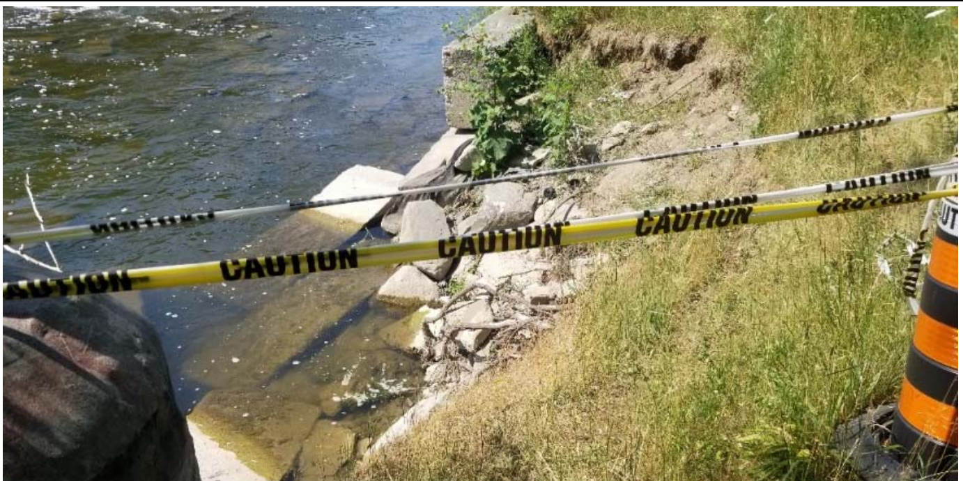
Photograph 2: View of displaced concrete blocks of the retaining wall at the location of the bank scour.
