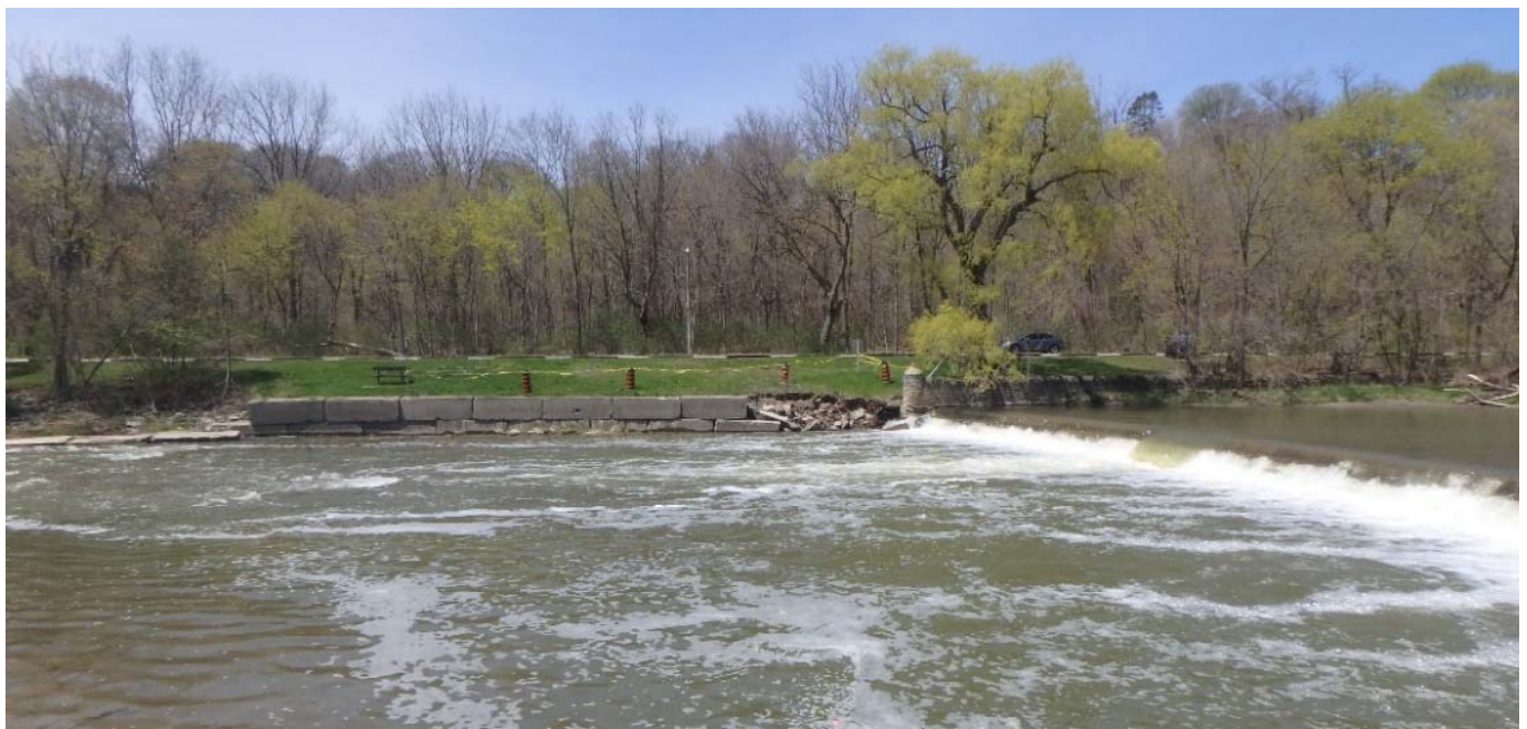
Photograph 1: View of the existing concrete block retaining wall and bank scour along the west bank.
